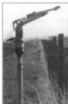
Valve on riser supported by underground concrete block.
